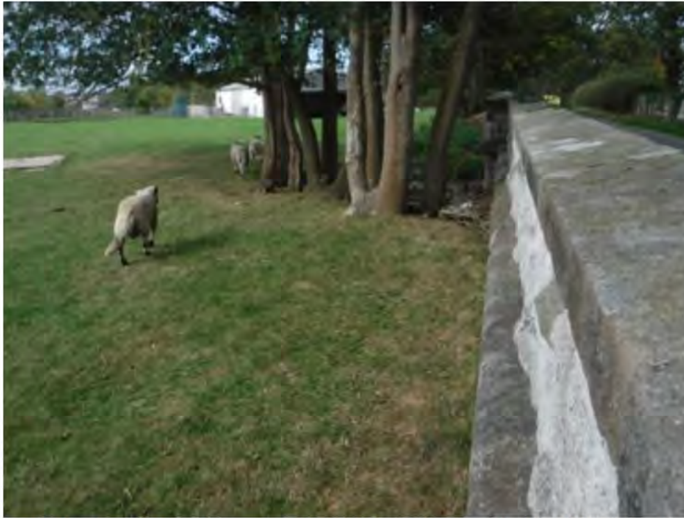
Photo No: 1 – Mature tree growth: Within of the proximity of the structure.
