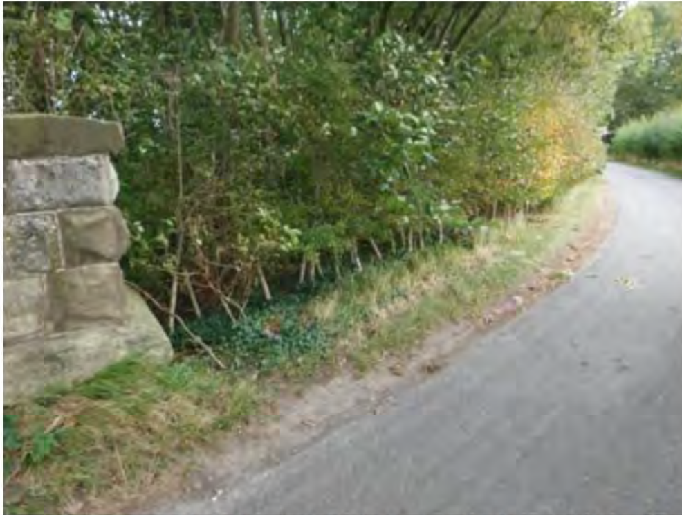
Photo No: 5 – Approach road fencing: Typical example of the condition at S/E end.
