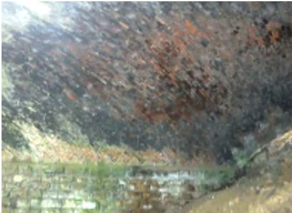
Photo No: 2 – Possible further deterioration: To the spalling brickwork areas.
