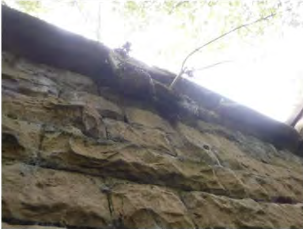
Photo No: 3 – Possible further deterioration: To the eroded stonework areas.
