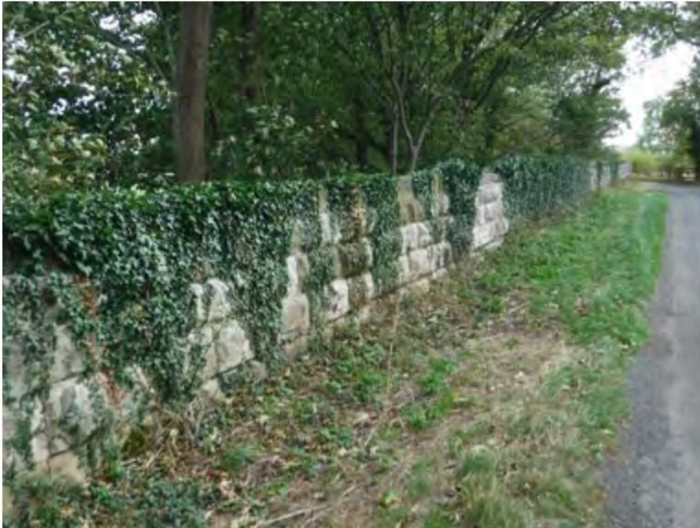
Photo No: 4 –Vegetation: Progressively getting worse.
